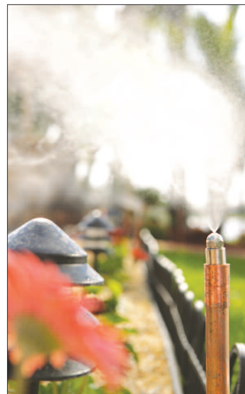
SWAT Mosquito Systems creates a mosquito-free barrier around your home, pool and backyard by installing a customized system of nickel-plated and stainless steel nozzles in order to kill mosquitoes and other biting insects.
